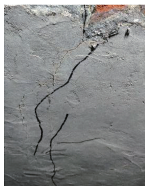
(a) 拱顶裂缝
